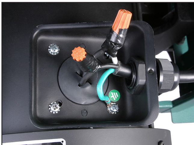
Figure 88. G0605X motor junction box.
